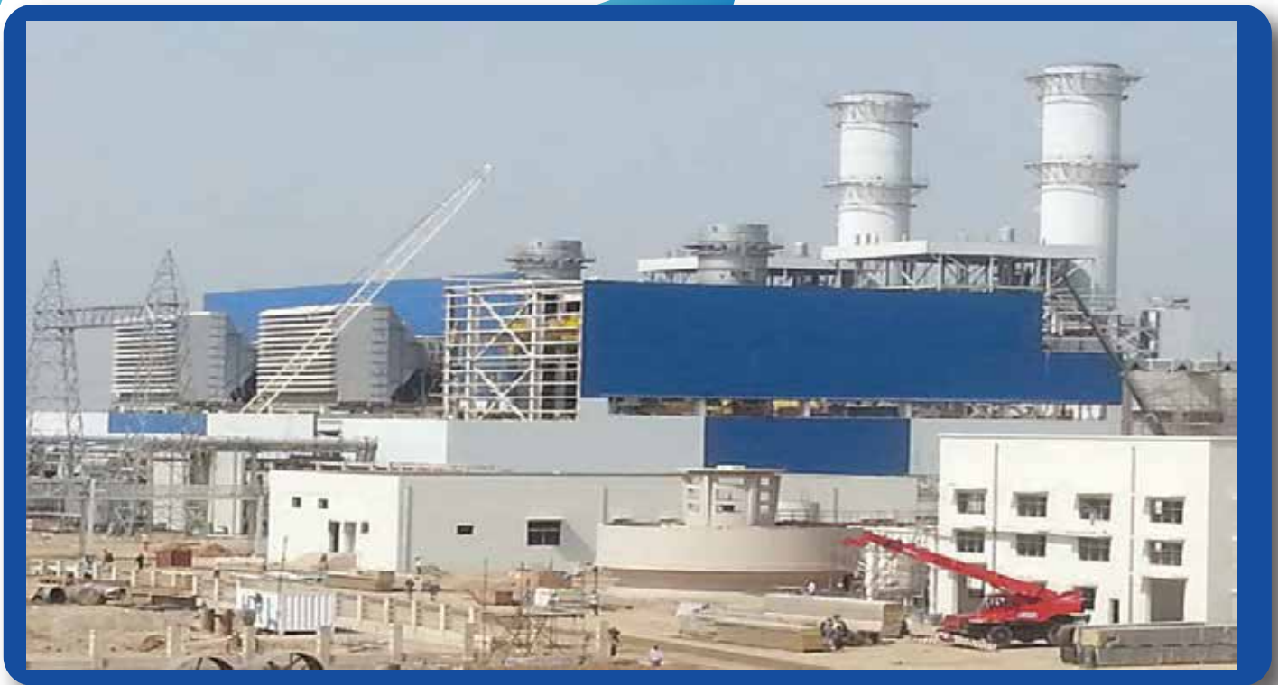
747 MW CCPP Thermal Power Project, Guddu, Pakistan. 2010 to 2014
